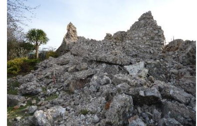
View of the wall after the collapse
