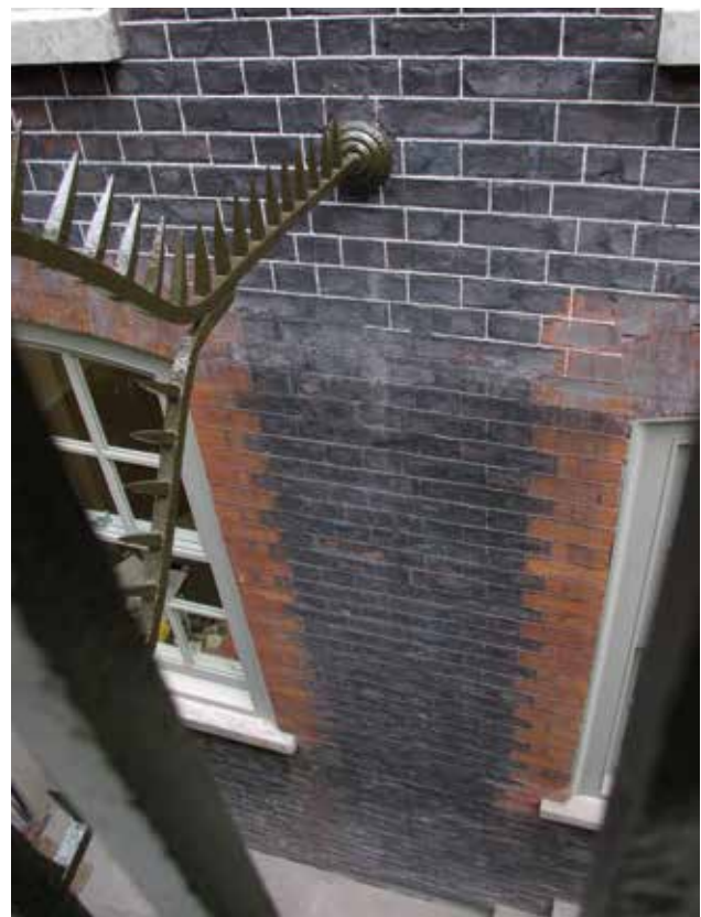
Fig 3 Detail of the restored front façade in 2008, showing original tuck pointing at lower ground floor level
