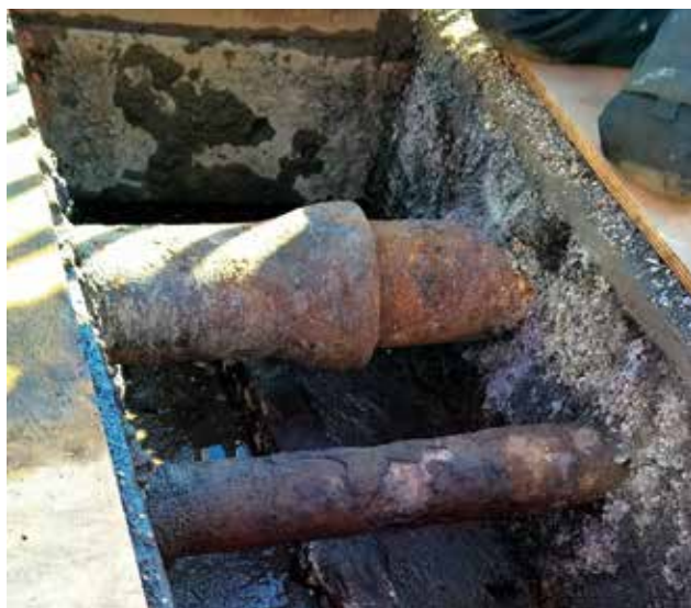
Fig 13 Trial hole investigations showing upstand to deck plates at right angles below the service pipes
