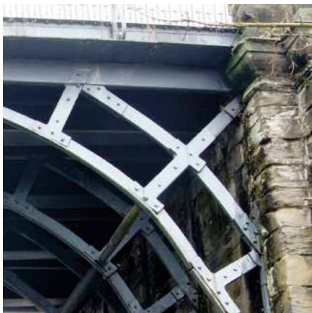
Fig 16 South span showing cracked ribs, gusset plates and inserted beams
