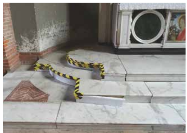
Fig 6 St John’s Chapel: water damage to wall and movement damage to paving
