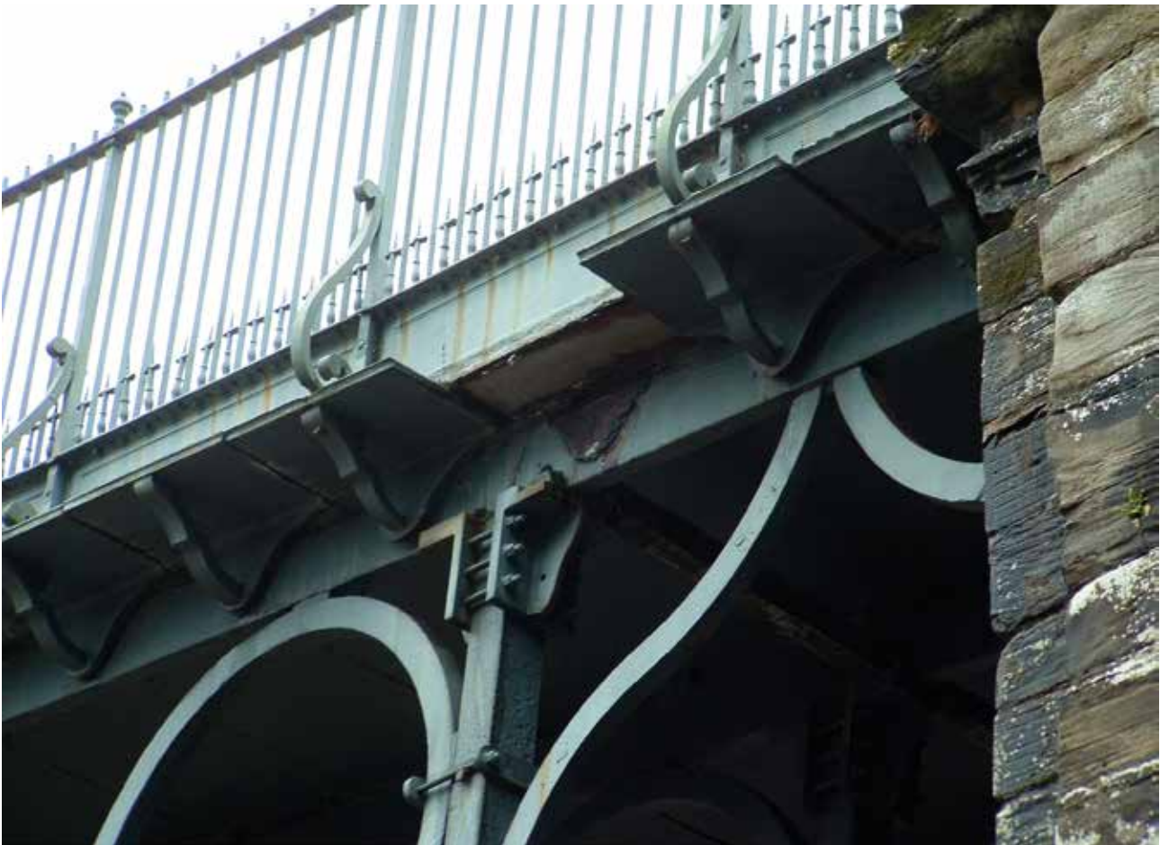
Fig 8 Saddles added at the top of the uprights to support the cracked bearers in 1927, following recommendations by the bridge trustees' surveyor Luther Griffiths, and missing deck plate end
