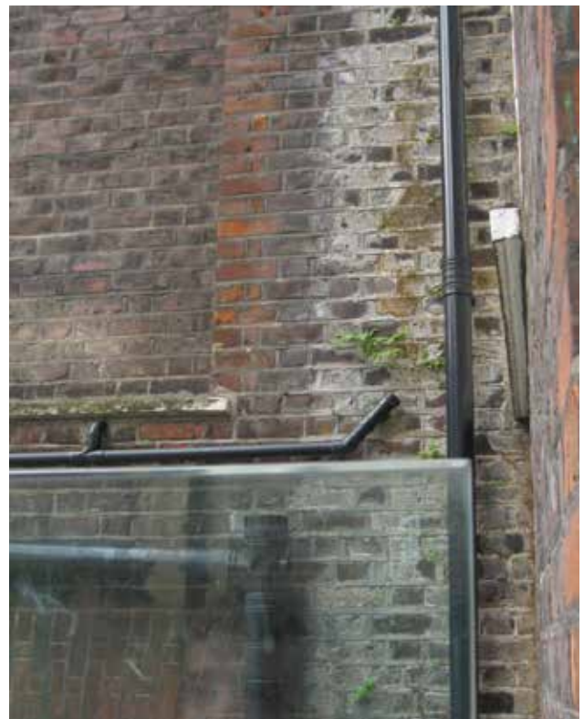
Fig 8 Existing salt contamination and plant growth on the rear façade brickwork, 2008
