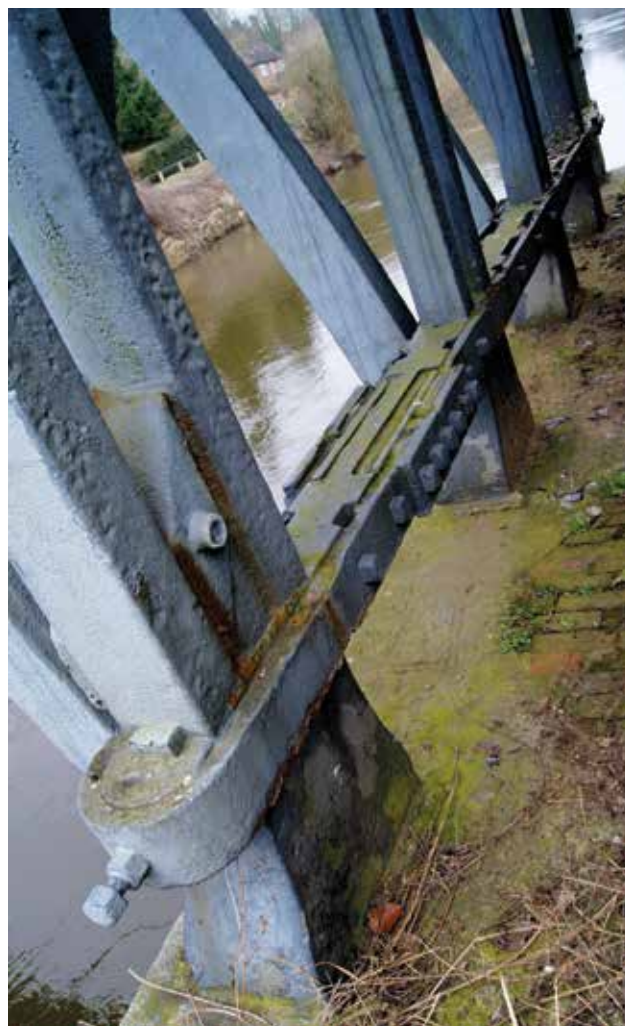
Fig 10 Photo of south bank steel straps and cast iron blocks installed after inspection by Sir Benjamin Baker in 1902 to restrain the feet of the uprights
