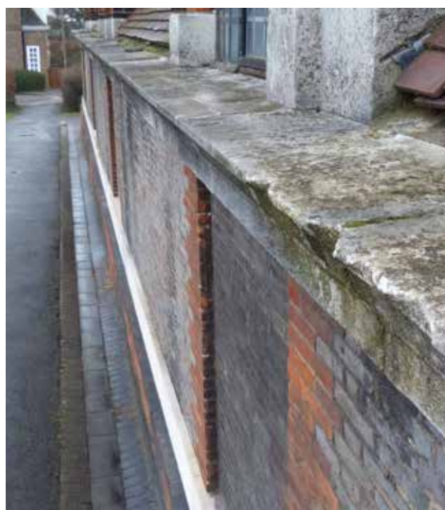
Fig 4 Detail of the cornice to the aisle walls with minimal fall to shed rainwater
