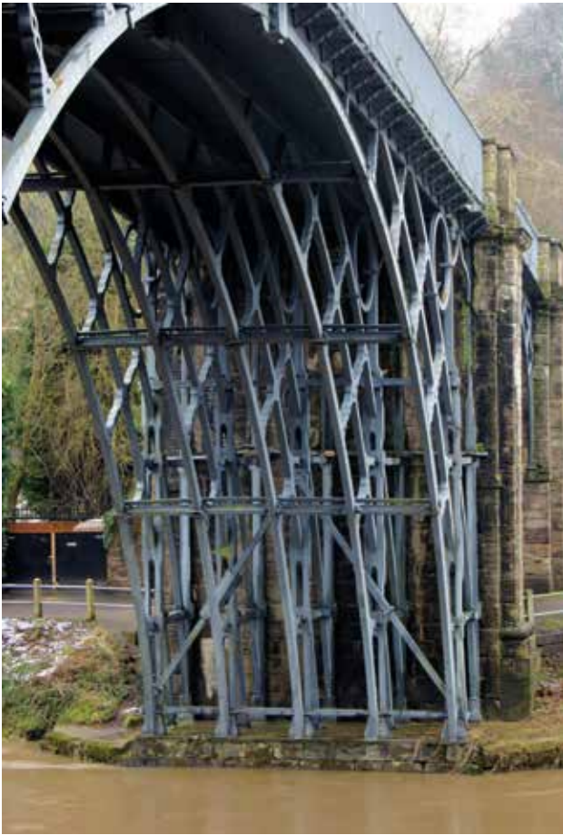
Fig 6 South bank showing horizontal strap just above the feet of the uprights and splint to diagonal bracing, both added following Sir Benjamin Baker's inspection in 1902
