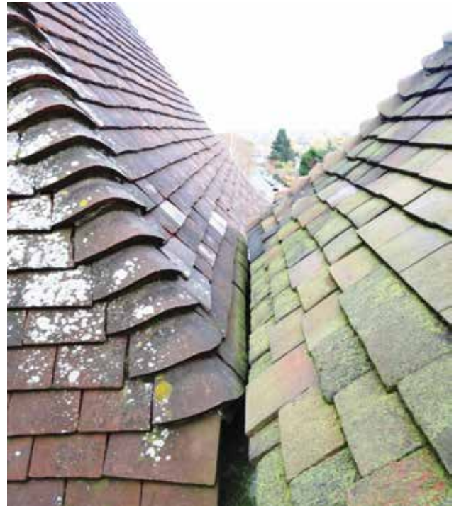
Fig 5 A difficult gutter to clean
