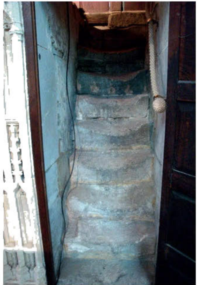
Fig 2 The internal staircase is much worn
