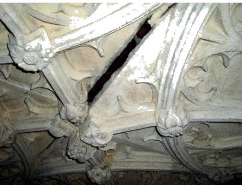
Fig 4 The crack in the vault
