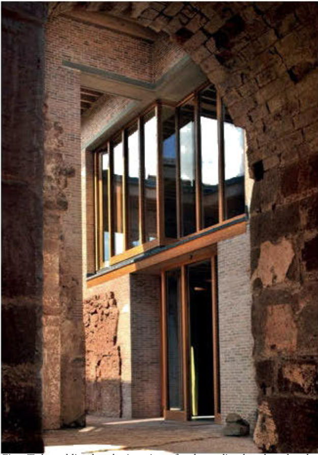
Fig 7 T-shaped lintel at the junction of early medieval, 15th and 17th century work
