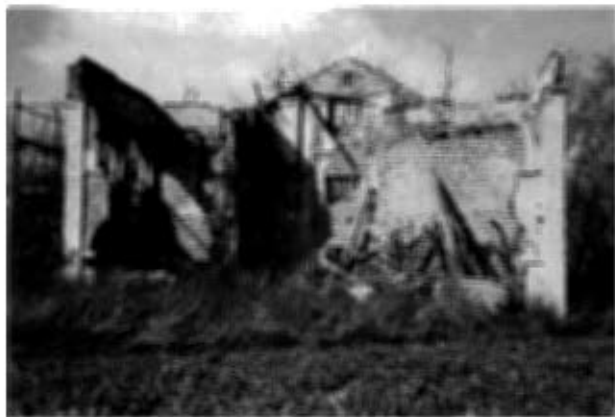
Figure 10 Stamford Grandstand, April 1995. Note patches of historic plaster; casement windows of 1766 and fallen remains of 1820 rendered parapet. (Author)
