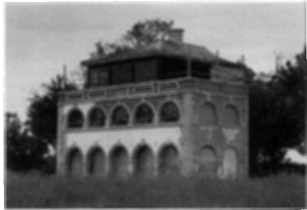
Figure 18 Coleford bricks instated in south façade being rendered; parapet being reinstated; new top storey with glazed openings in steel frame and swept copper roof constructed over timber frame, June 1996. (Author)
