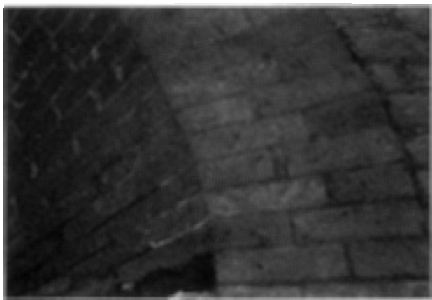
Figure 9 Detail from the face of the large-span, canted semi-circular gauged arch at 64 Breestraats, Leiden, showing striations made by the use of the steenschaaf.
