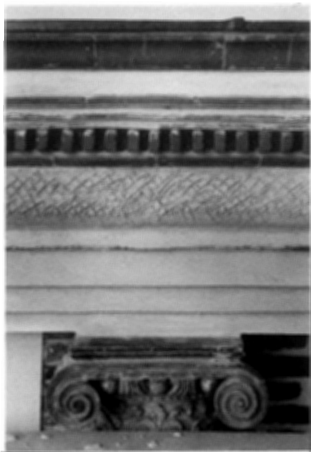
Figure 12 Detail of Ionic entablature with profiled terracotta and plaster undercoats.
