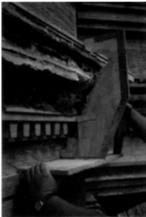
Figure 26 Cornice to West Courtyard elevation. The early-19th-century Roman cement dentils survive, but the rest of the profile needs major building up.
