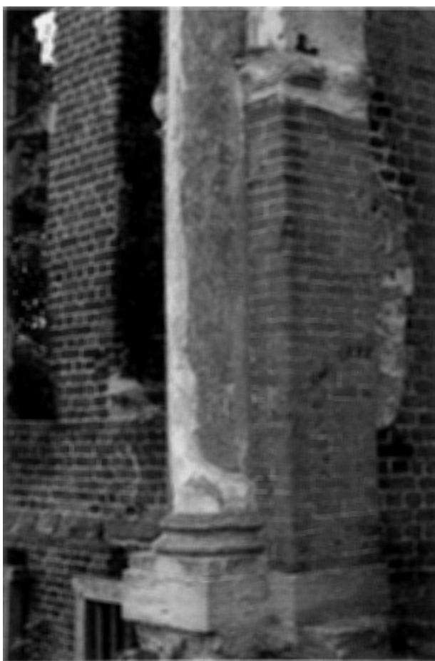
Figure 2 Part of the early gauged brickwork at Houghton House, Ampthill. This gauged work is part of a Renaissance-styled alteration attributed to Inigo Jones.
