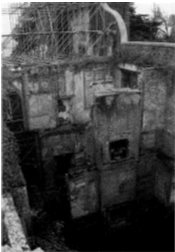
Figure 6 View over the West Range in 1993, with scaffold shoring to gable end wall of South Range.
