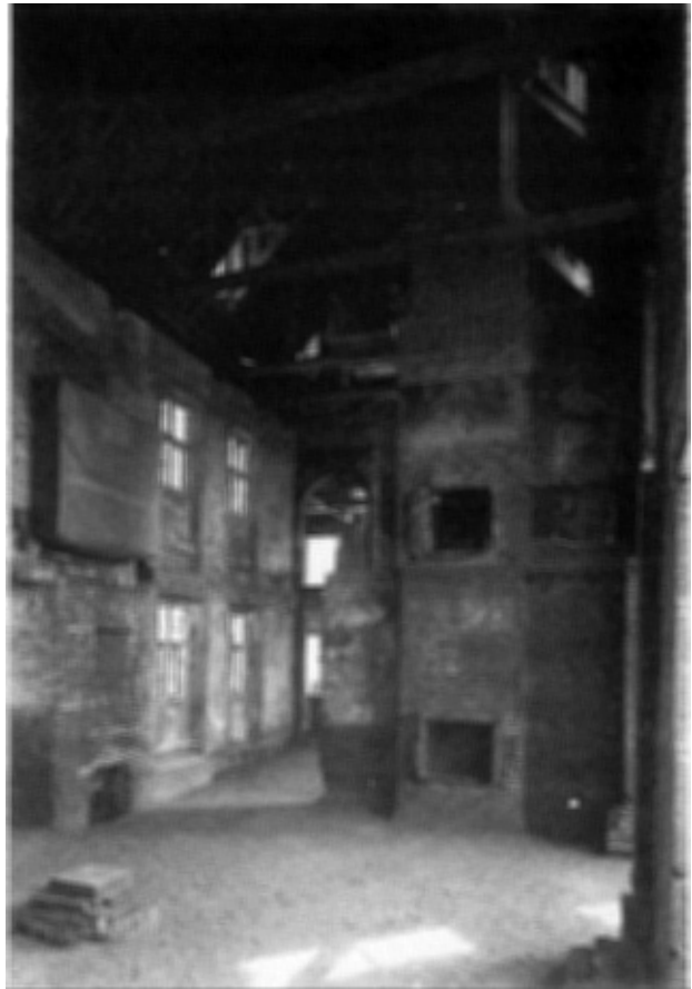
Figure 29 Interior view of the West Range after completion of the external envelope restoration. Compare with figure 6 .
