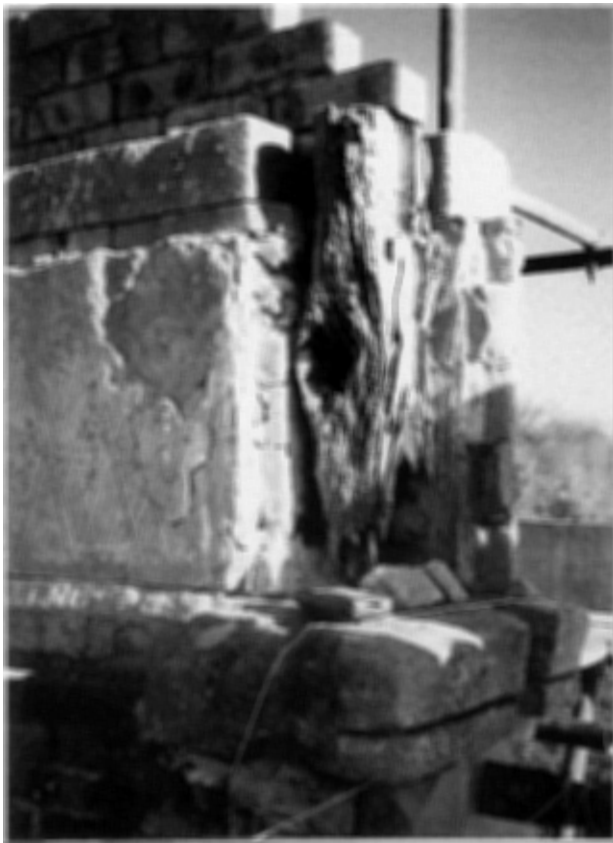
Figure 14 Wizenod timber is all that remains of the second floor roof structure, November 1995. (Author)
