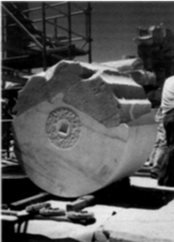
Figure 3 Restoration of lost stone to a column drum, before cutting of flutes. The new marble will be toned down to harmonise with the appearance of the original, though still readily distinguishable.
